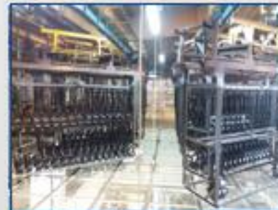
Power & Free System (covering the complete plant layout)
